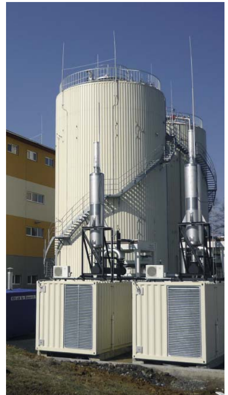
Digester vessel of the Benešov plant; the plant is currently in trial operation and is to be handed over to the client in mid-2009
